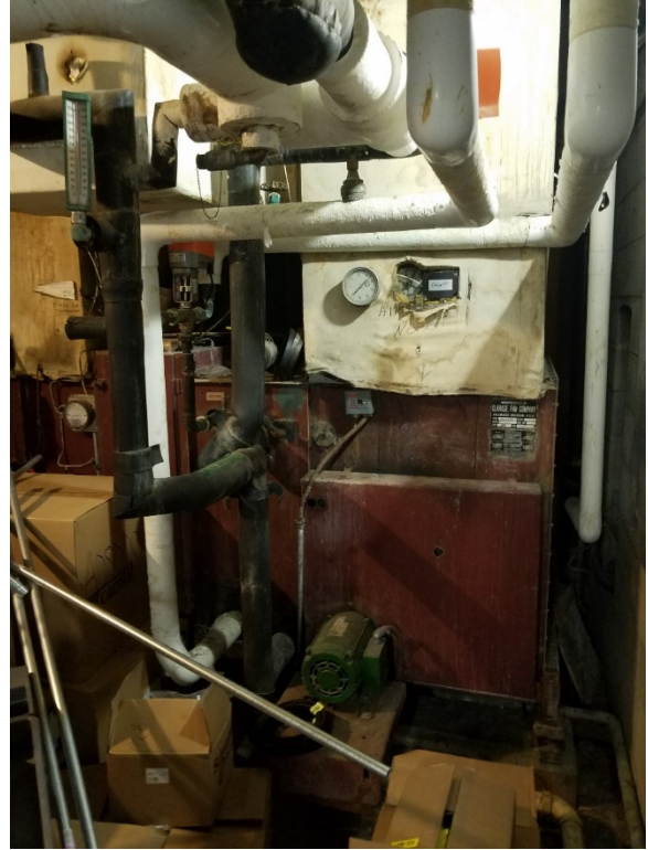
Old Air Handler
