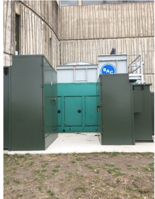
Terrace Dining Hall - medium voltage service upgrade
